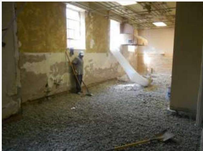
Sept. 27—The kitchen after several days of demolition, including jack-hammering the entire floor.
